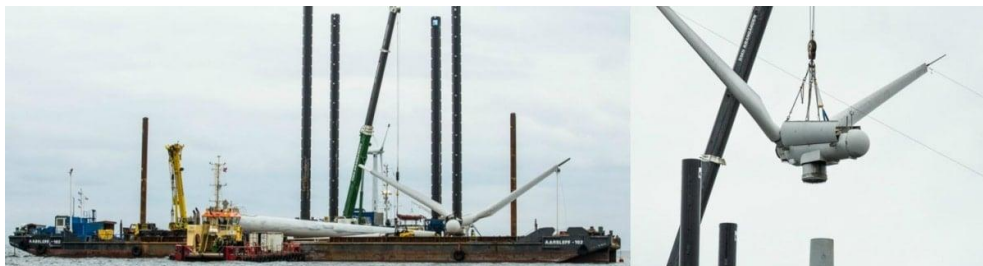
Figure 2-3 Wind turbine removal via bunny ear configuration and the vessels involved during Vindeby offshore wind farm decommissioning 3 .
